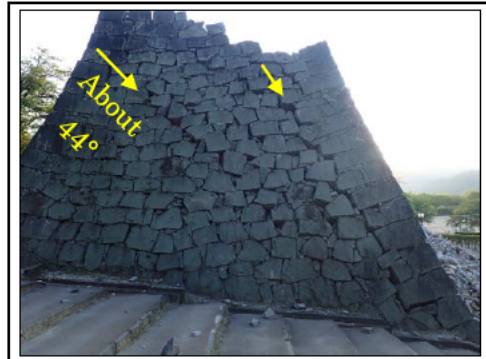
Damage of stone walls at Kumamoto Castle by the 2016 earthquake: Multiple failure modes, detaching of stone walls and active failure of the backfill ground could be seen (photo provided by Dr. Kikumoto)
